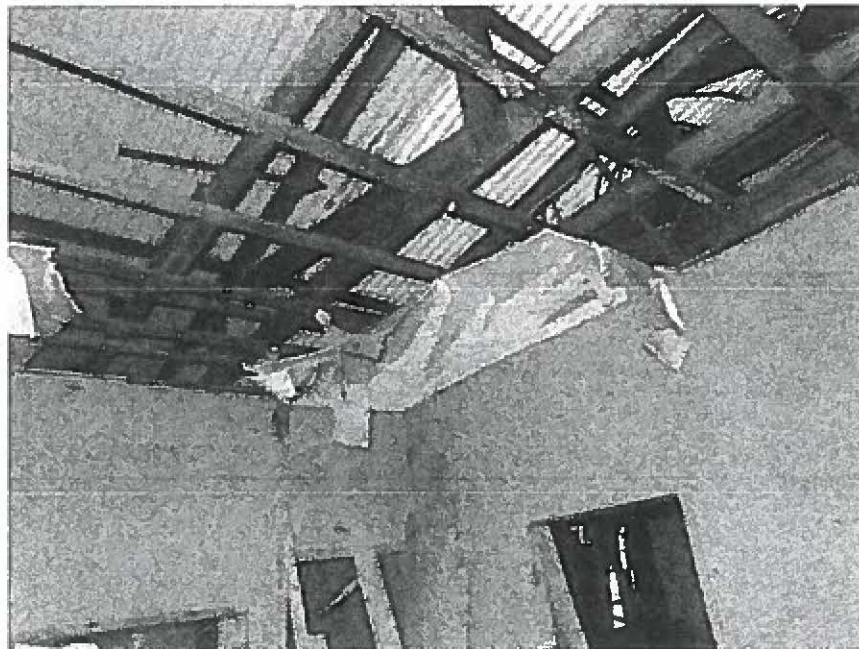
Photo 18 – Evidence of rot and corrosion due to leaking roof
