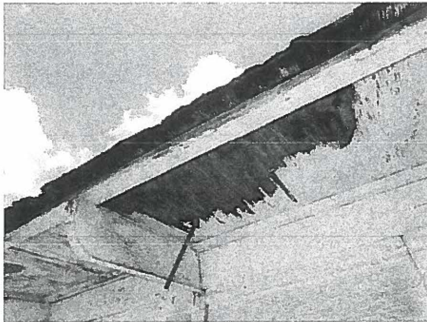
Photo 4 – Typical deteriorated plywood sheathing
