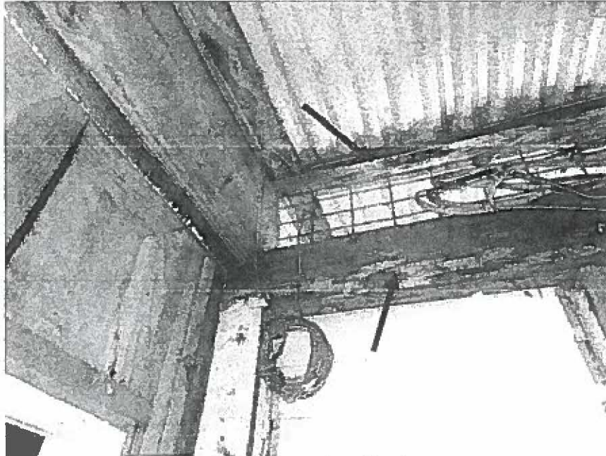
Photo 17 – Severe termite damage
