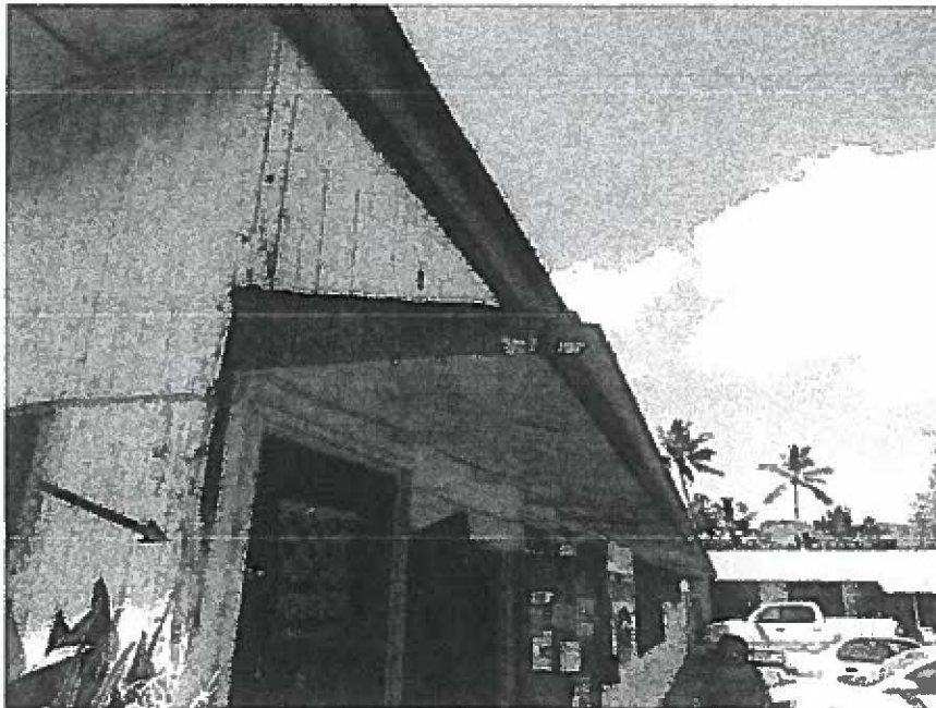
Photo 6 – Typical deteriorated 1x6 plank (near entrance)
