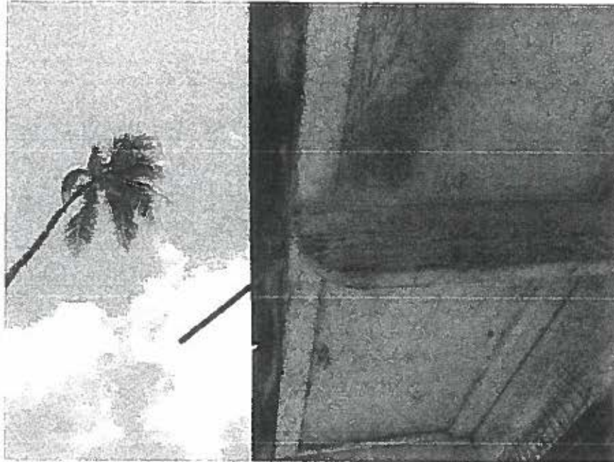
Photo 1 – Typical termite damage to roof rafter at eave
